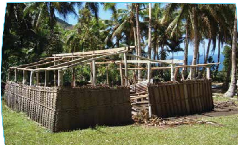
Damage to a house from Tropical Cyclone Gene, January 2008.
