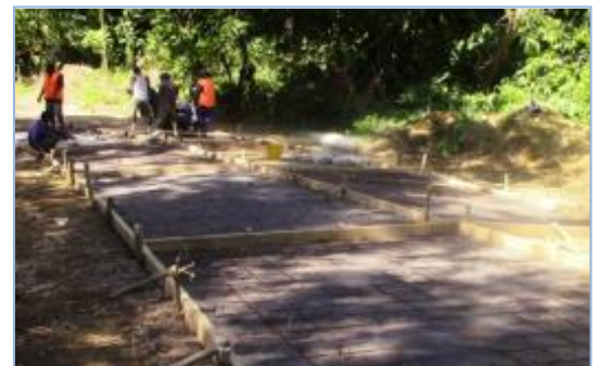
Work conducted by PWD to construct concrete tracks and train local labour (Ian Lercet/PWD 2013)
